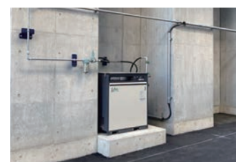
Model: SMS8ESD (Outdoor installation) Location: Manufacturing Plants
