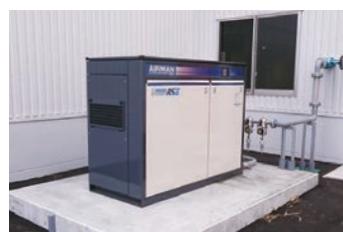
Model: SMAD22SD (outdoor installation) Location: Manufacturing plants
