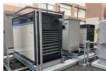
Model: SMAD55VD (outdoor installation) SMAD22VD (outdoor installation) Location: Research laboratories
