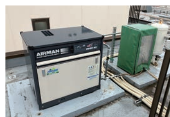
Model: SMS4ESD (Outdoor installation) Location: Manufacturing Plants
