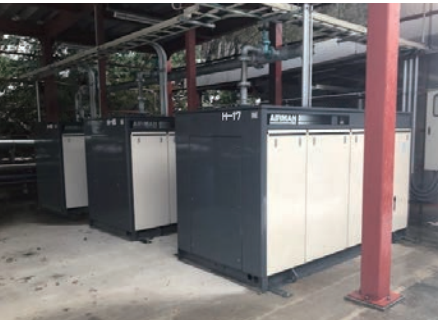
■ Model: MWS160S ■ Location: Casting Plant
