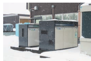
Model: SMAD55VD (outdoor installation) Location: Manufacturing plants
